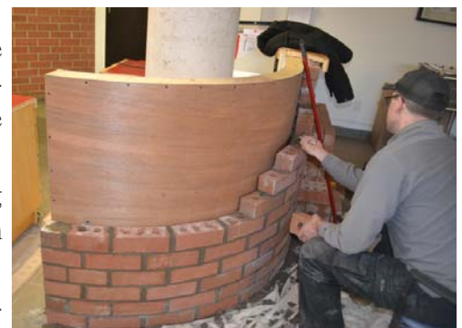
Ongwanada's carpenter installing the new accessible reception desk at Resource Centre in January
